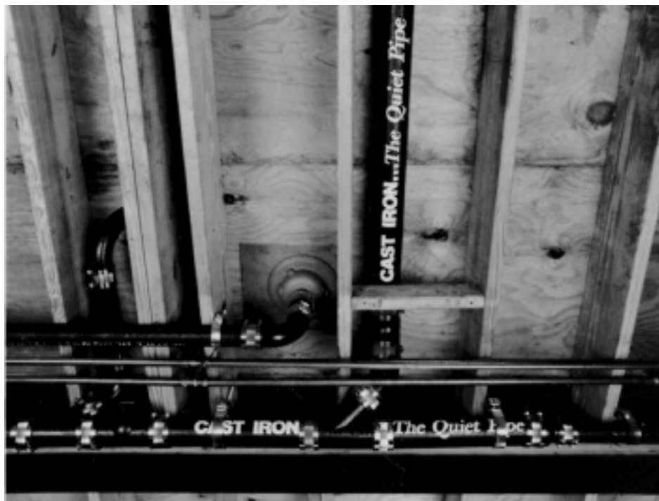
Figure 1—Cast Iron in Residential Application.
